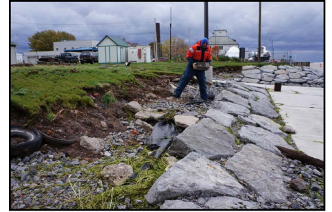
Brian Haas inspecting a section of shoreline with major erosion showing the loss of lawn from the high waters.
