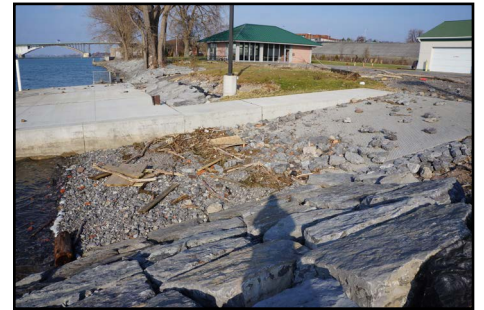
Stone deposited in the boat launch from the storm, filling most of the ramp with gravel of various sizes.
