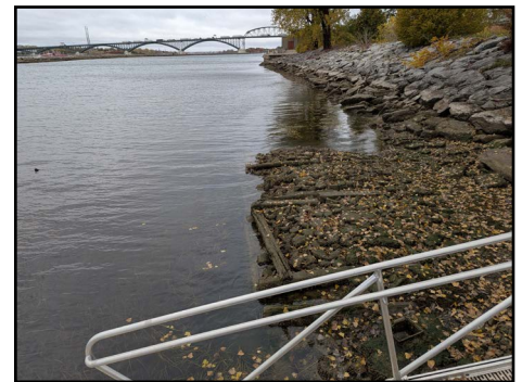
Cribbing exposed during the October 23 rd seiche.
